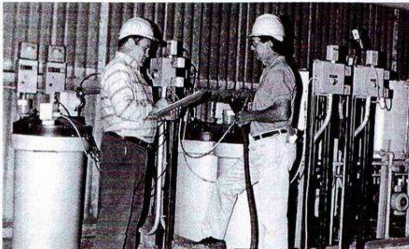
A chemical feed system injects alum and polymer into the incoming water for coagulation and flocculation.
